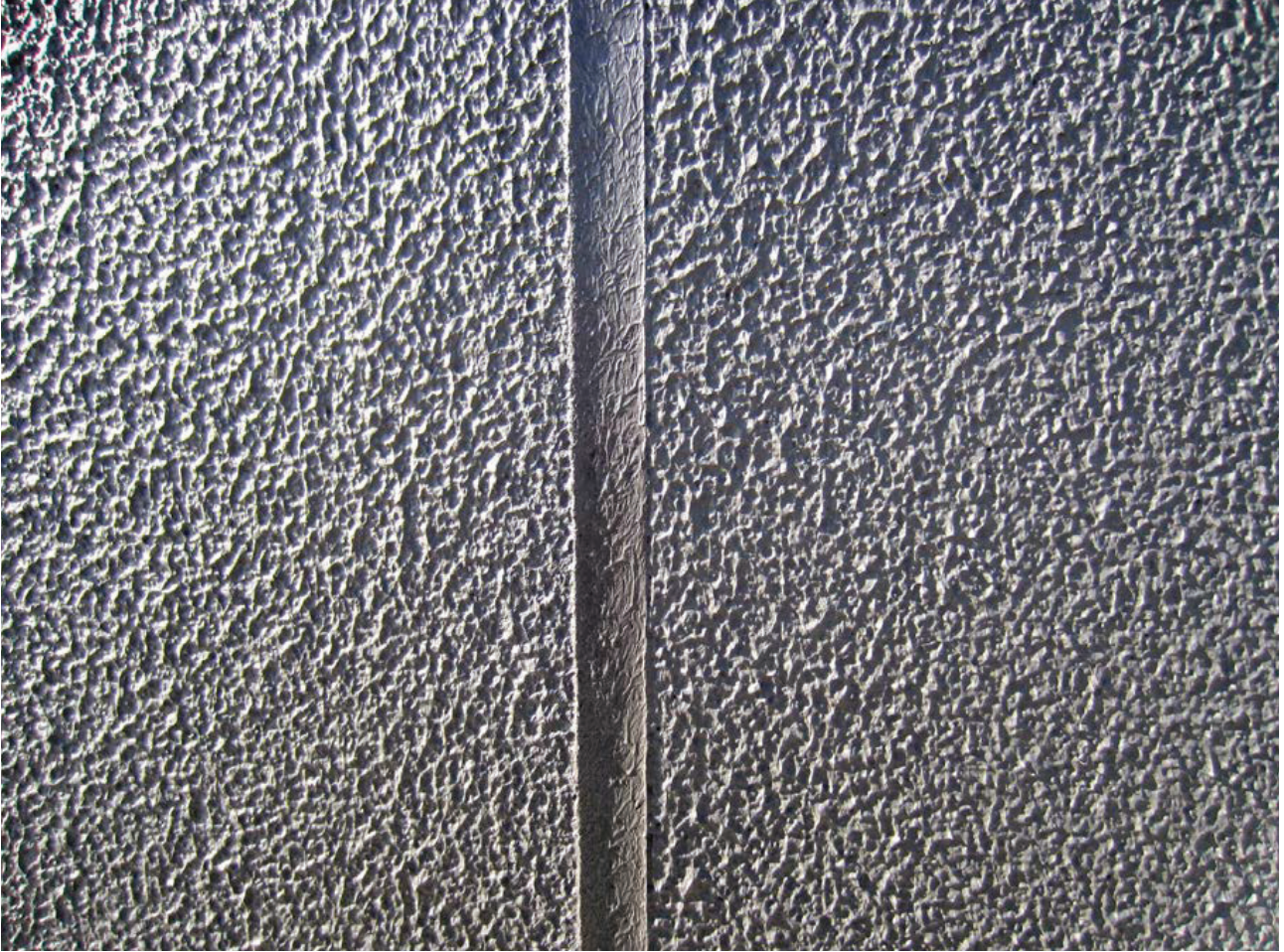
PHOTO SHOWING WESTERN WALL – DARK COLOUR 5MM THICK RENDER WITH 5MM WIDE JOINT APPLICATION ON DINCEL-WALL
